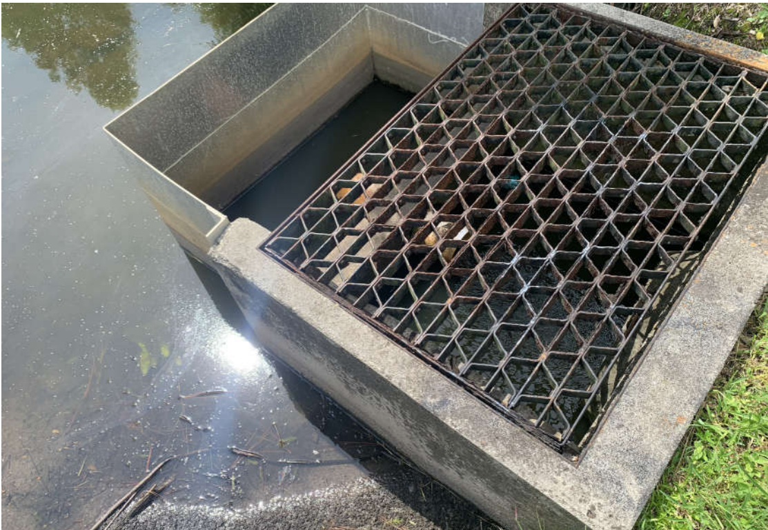
Overflow Structure Basin 5
