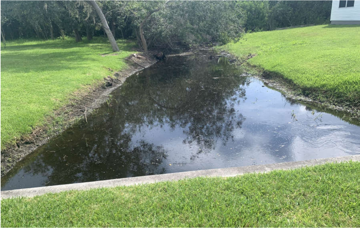
Erosion at Southern Spillway
