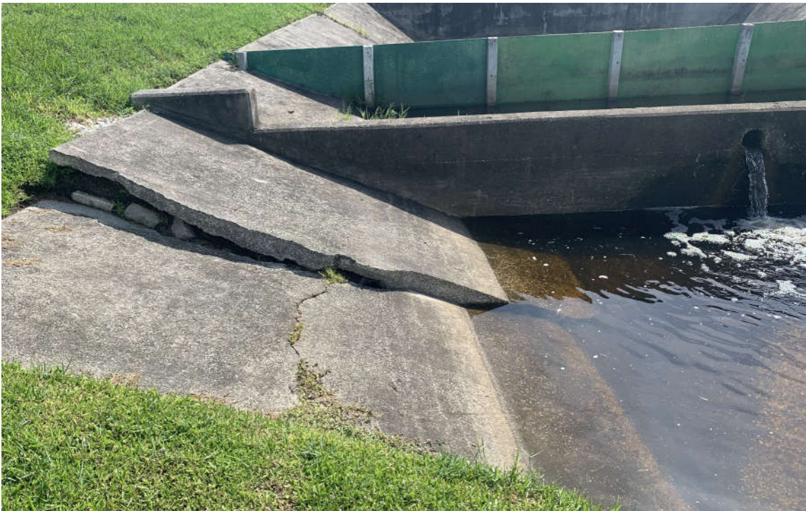
Cracked Concrete @ Northern Spillway
