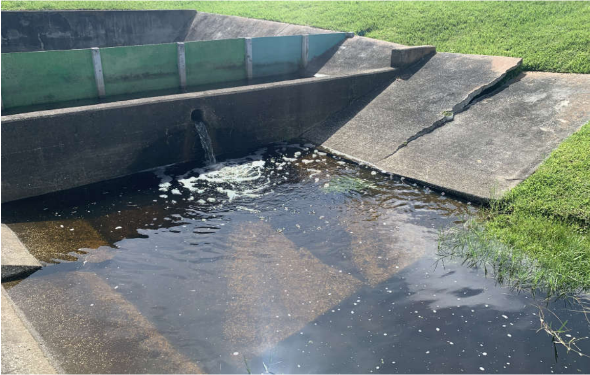
Cracked Concrete @ Northern Spillway
