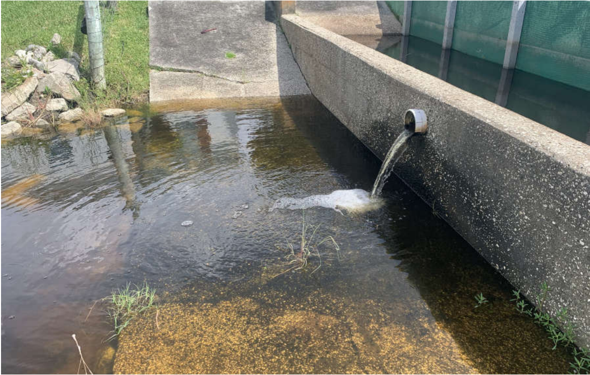
Southern Spillway missing Debris Trap, Cracking of Concrete
