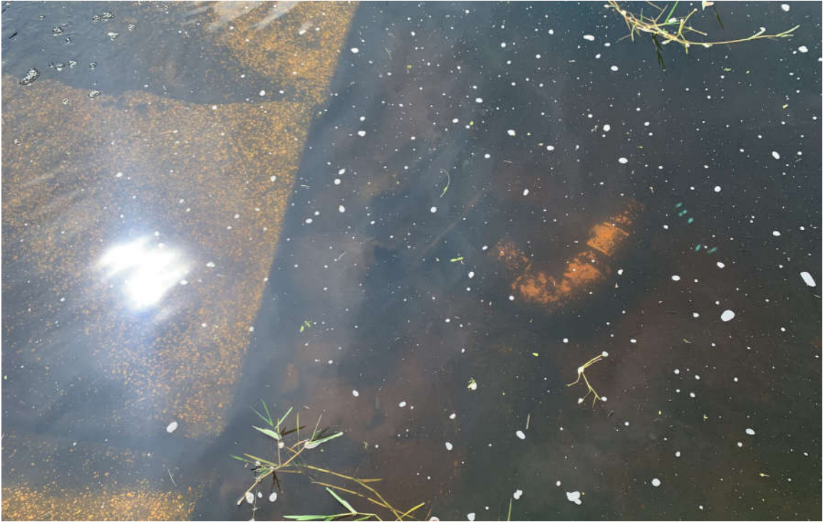
Broken Beehive Debris Trap @ Northern Spillway
